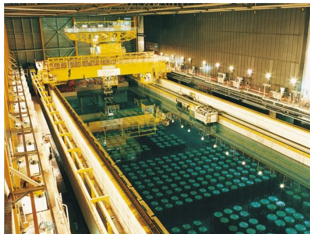
Modern spent fuel cooling pond
